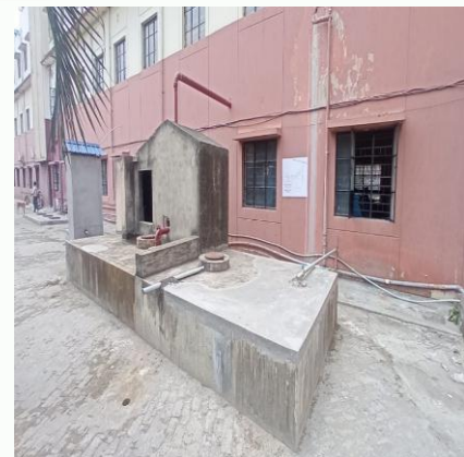
Rooftop Rainwater Harvesting
